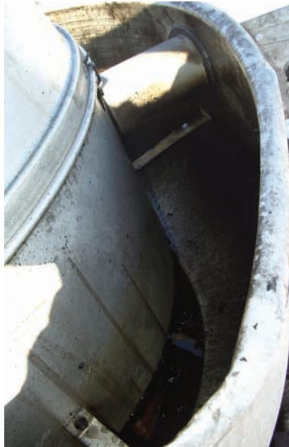
Typical extractor, 3 months since prior cleaning. Notice the accumulation of grease liquids in the bottom of the extractor.
