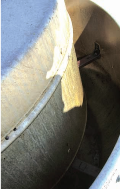
Applebee's Murrieta, California, extractor with the new system, 6 months since prior cleaning. Notice the bottom of the extractor has only a light film of grease effluent, and there is no accumulation of liquid grease in the bottom of the extractor.
