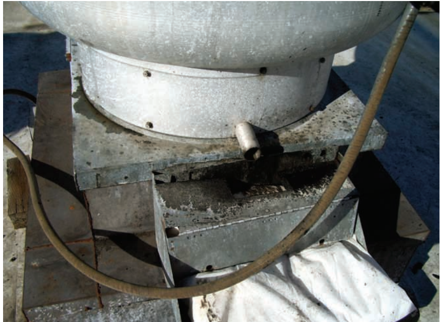
Another typical extractor with overflow discharge, 3 months since prior cleaning. Notice the overflow has spilled onto the roof area around the extractor.
